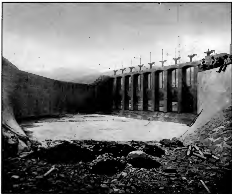
HEADGATE ON MAIN CANAL FROM TRUCKEE RIVER
